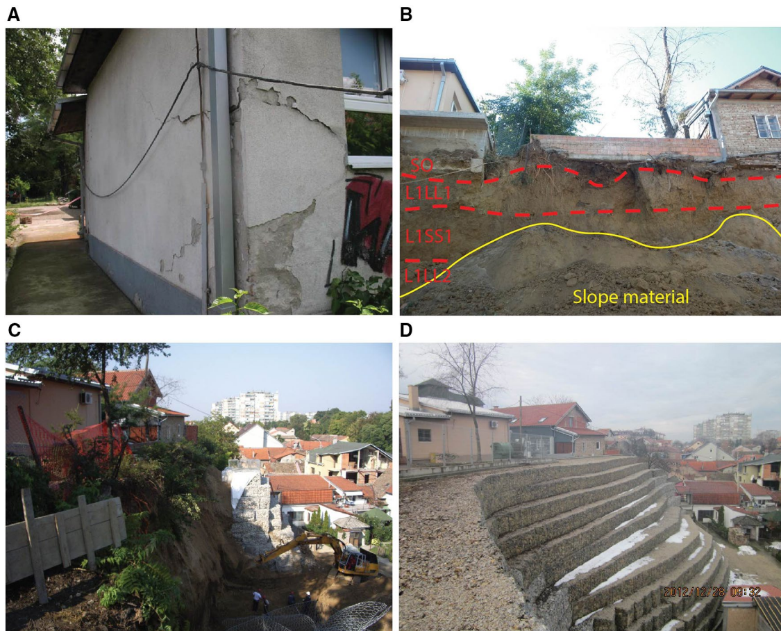
Fig. 8 a The kindergarten facility before the 2010/2011 landslides. b View from the base of the slope after landslide event in 2010. c Rehabilitation works following the landslide event in 2010. d Installation of retaining walls at the end of 2012 (Photo: Mladan D)
